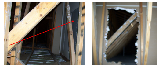
Allowed self-closing door with automatic latch in the draftstop wall of an attic.
